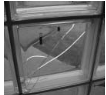
Cracking due to incorrect expansion joint
